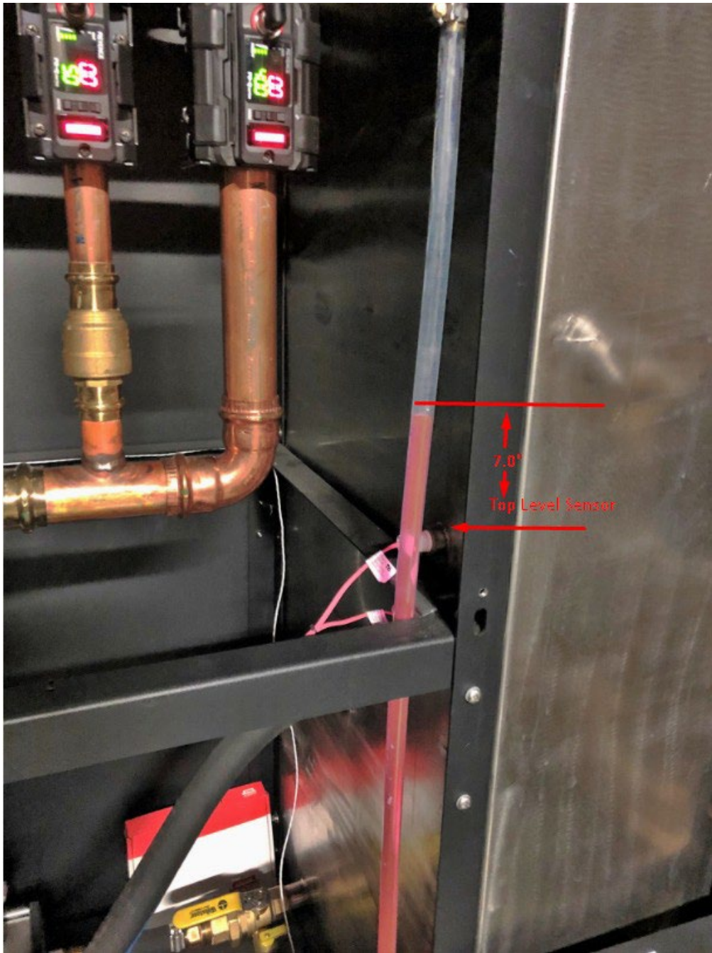
The coolant level is checked in the plastic hose on the right side of tank, and it should be about 6.0" to 7.0" above the top level sensor.
