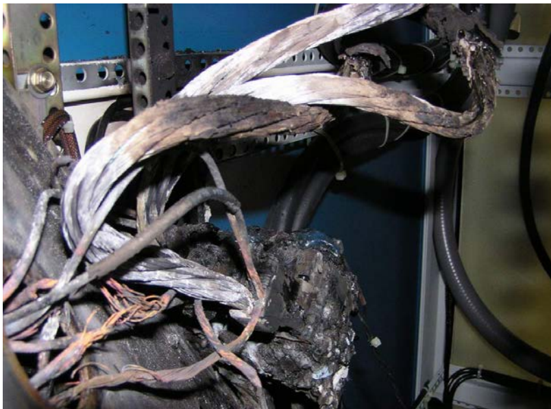
Example of an AC Mains catastrophic failure
